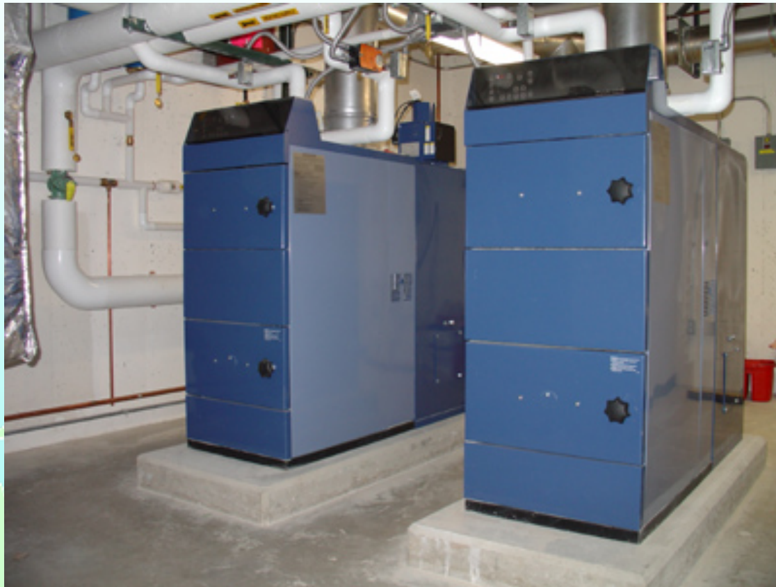
Two Tarm 4.0 40 kW Boilers
